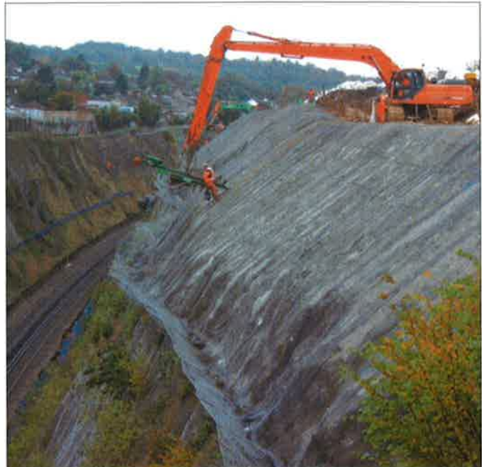
Installation of soil nails through Deltax mesh, laid on existing slope face
